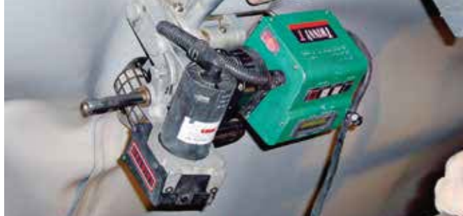
TWINNY T, with convenient cross-handle, at work overhead welding in a tunnel.
